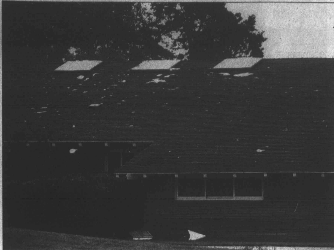
Open-air skylights ... Homeowner Todd Lockaby probably had a little too much sky showing through his skylights after Sunday night's hailstorm in Tahoka, as all three were shattered by the massive hailstorm that slammed into the area.
