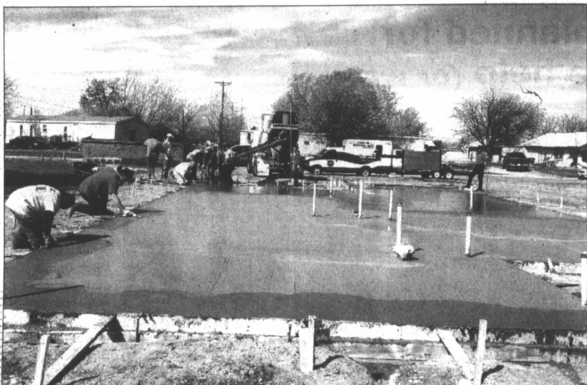
Foundation for Butterfly Blessings ... The foundation for the "Butterfly Blessings for Laela Duran" home building project was poured last week. This weekend is a major work weekend at the site at 1318 Ave. K. Volunteers, both professional and non-professional, are expected to help erect the home, working Thursday through Sunday.
