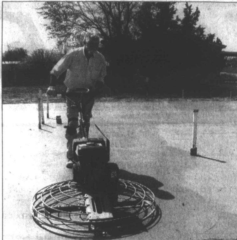
Mitch's trowel ... Mitch Raindl uses his troweling machine to finish setting the concrete in the foundation at the Duran home building project Saturday. (LCN PHOTO by Juanel Jones)
