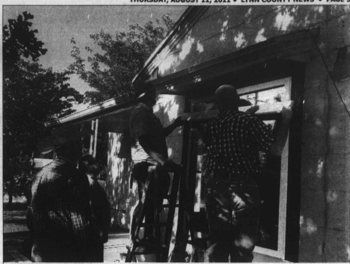
Helping hands... The H.O.M.E. (Hands on Mission Evangelism) group met on Saturday, August 6, at the home of Mr. and Mrs. Ynes Aleman, replacing windows and installing window air conditioner units. Pictured here from left are Mike Huffaker, Danny Hart, Ty Askew and Alton James. (LCN PHOTO by Pam Elrod)
