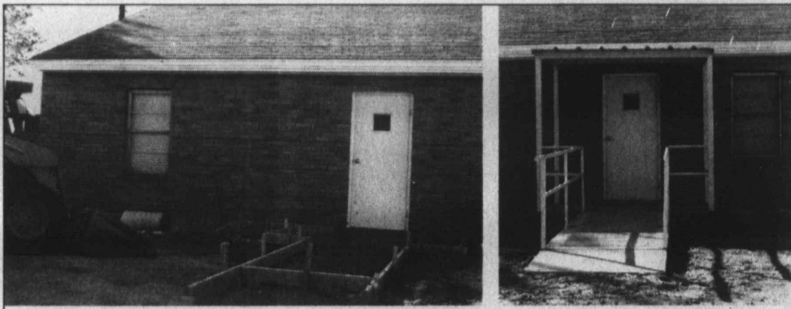
Improvements ... First Baptist Church in Wilson has recently improved the back entrance to their fellowship hall by making it more handicapped accessible, and added a porch roof as well. These pictures show the work in progress, and the results of the hard work.
