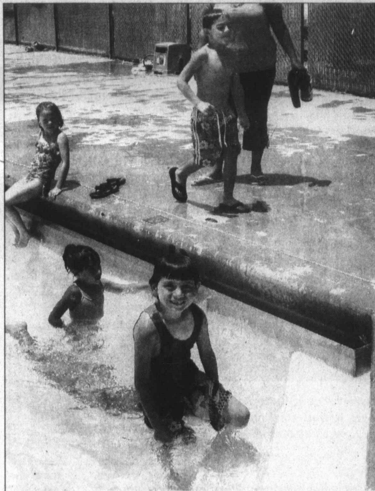
Updated pool ... Children swimming and playing in the Tahoka City Pool probably don't notice it much, but city officials are proud of the new stainless steel gutter that replaced the broken tiles around the inside edges of the pool, making the pool a safer place for pool patrons. The pool is open Wednesday-Sunday from 12:30-5:30 p.m., at 1715 South 8th Street.
