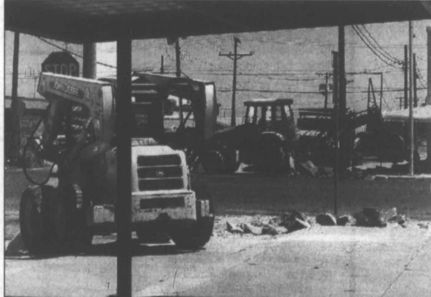
Handicap access ... New handicap access ramps are being placed throughout Tahoka on Lockwood and Main Streets, as the State contracted out to have the work done. Workers in this picture are at the corner of Main and Harper Street (adjacent to The Lynn County News) taking out the old ramps which are no longer up to code, and replacing with wider ramps on two sides of each corner curb that feature a special pebbled texture for statewide standards for the blind. Workers said they hope to complete the Tahoka ramps in about three more weeks.
