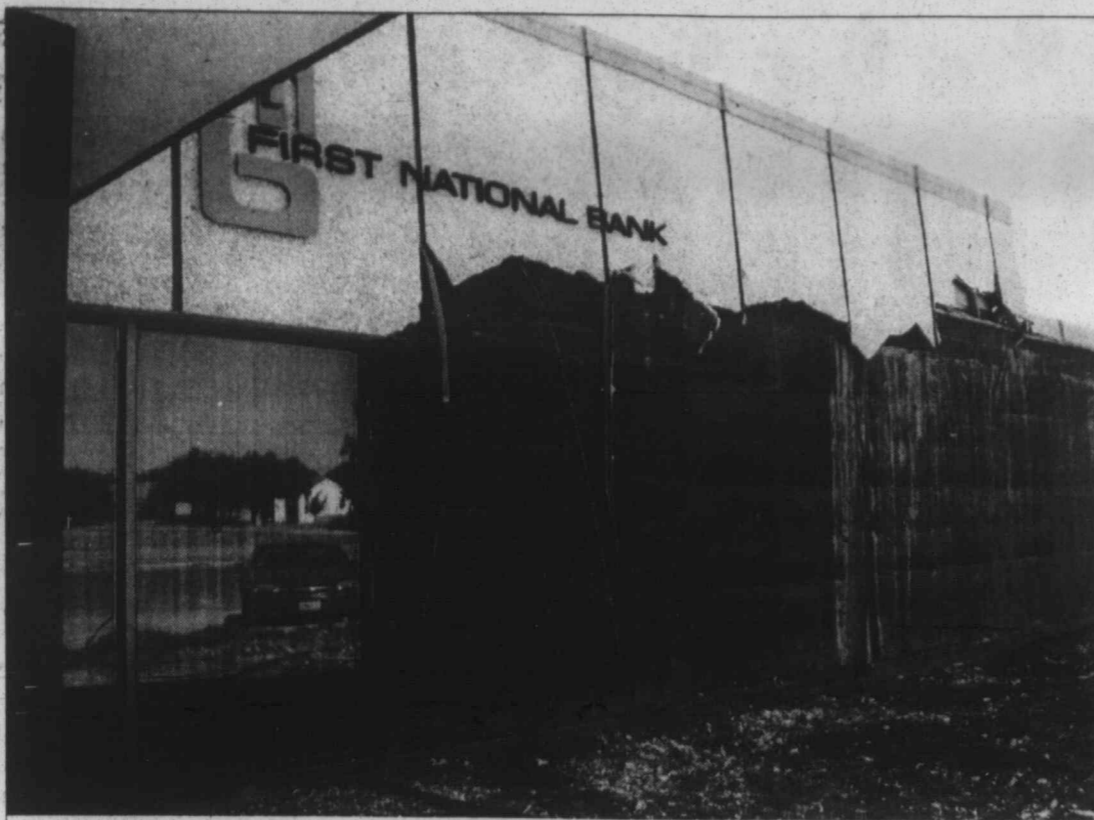
New look coming ... First National Bank began undergoing exterior renovation last week, removing the white stucco/rock exterior to replace with a new brick finish. Currently in their 100th year of service, FNB built this building in 1971.
