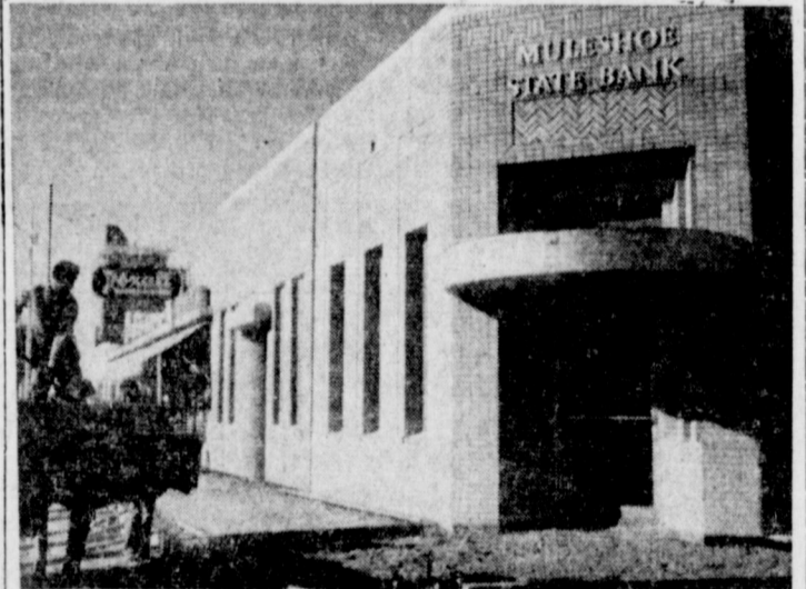
PROGRESS ON MAIN STREET — Muleshoe State Bank patrons noticed last week that there was construction going on in front of the bank. Workers were doing the groundwork for the installation of a four-foot clock to be installed on the corner of Avenue C and Main Street. The clock, which will revolve, will show the temperature on one side and time on the other. It should be erected by the end of this week, barring further bad weather. (Journal Engraving)
