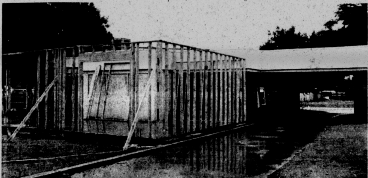
WILSON BANK EXPANDS — Wilson State Bank's Tahoka Branch office is expanding, with construction underway to add approximately 1,000 sq. ft. of space to the building located at 1900 Lockwood. The project is expected to be completed by Sept. 1, and will include expansion of the lobby area as well as an additional office area. (LCN PHOTO)
