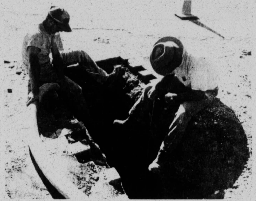
WHAT'S DOWN THERE? - Mostly mud, as workers dig down several feet to the city water lines, replacing the old pipes with new water lines. Here, they are using suction equipment to keep the area cleared in the deep hole. The city project is being funded through TCDP grant money, with new lines being placed from Kington to Ave. P on South 1 st Street, and from S. 1 st to S. 8 th on Ave. L. This site is at the corner of Main and South 1 st . (LCN PHOTO)
