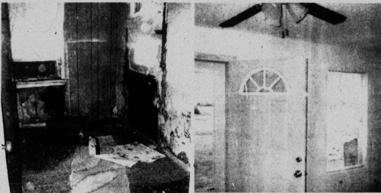
BIG CHANGES - Lending Hands, a volunteer organization that cleans up and repairs homes, has completed renovations on the home of Helen Bookman of Tahoka. The renovations include a new roof, windows and doors, new sheet rock and wiring and fresh paint inside and out. These before and after photos show the difference the volunteers made on the inside of the home.
