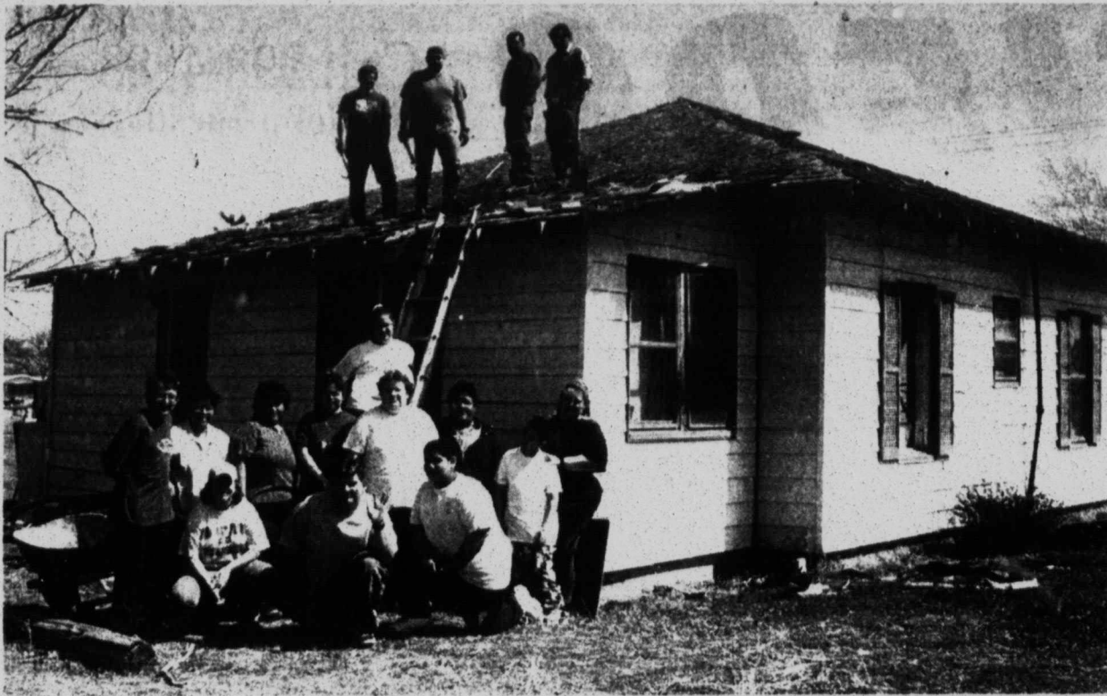
LENDING A HAND - This house at N. 5th and Ave. O in Tahoka is getting a new roof and the yard cleaned up, thanks to the help of 23 volunteers who are helping Urban Garcia with the project. Garcia, who owns the home, provided the roofing materials and George Sepeda, with the help of Sara Alvarado at South Plains Community Action, enlisted the aid of others. The idea originated at the local community action organization, but Mrs. Alvarado said no funding came through the agency. Sepeda calls the volunteers "A Lending Hand" and hopes that others will offer volunteer help with other projects. To find out more, contact the local agency. Shown here working Saturday morning are (on the roof) Roger Locke, Urban Garcia, Jessie Alvarado, George Sepeda; (standing) Robert Cruz, Aurora Cruz, Ricarda Salinas, Sara Alvarado, Tawanna Norris, Odelia Sastre, Cris Flores, Charline Flores, Keely Harcrow (on ladder); and kneeling, Kerri Cowley, Jimmy Speckman and Joshua Sastre. Special thanks is given to Rick Cloe and community service workers who picked up trash in the alley following the weekend's work. (LCN PHOTO)
