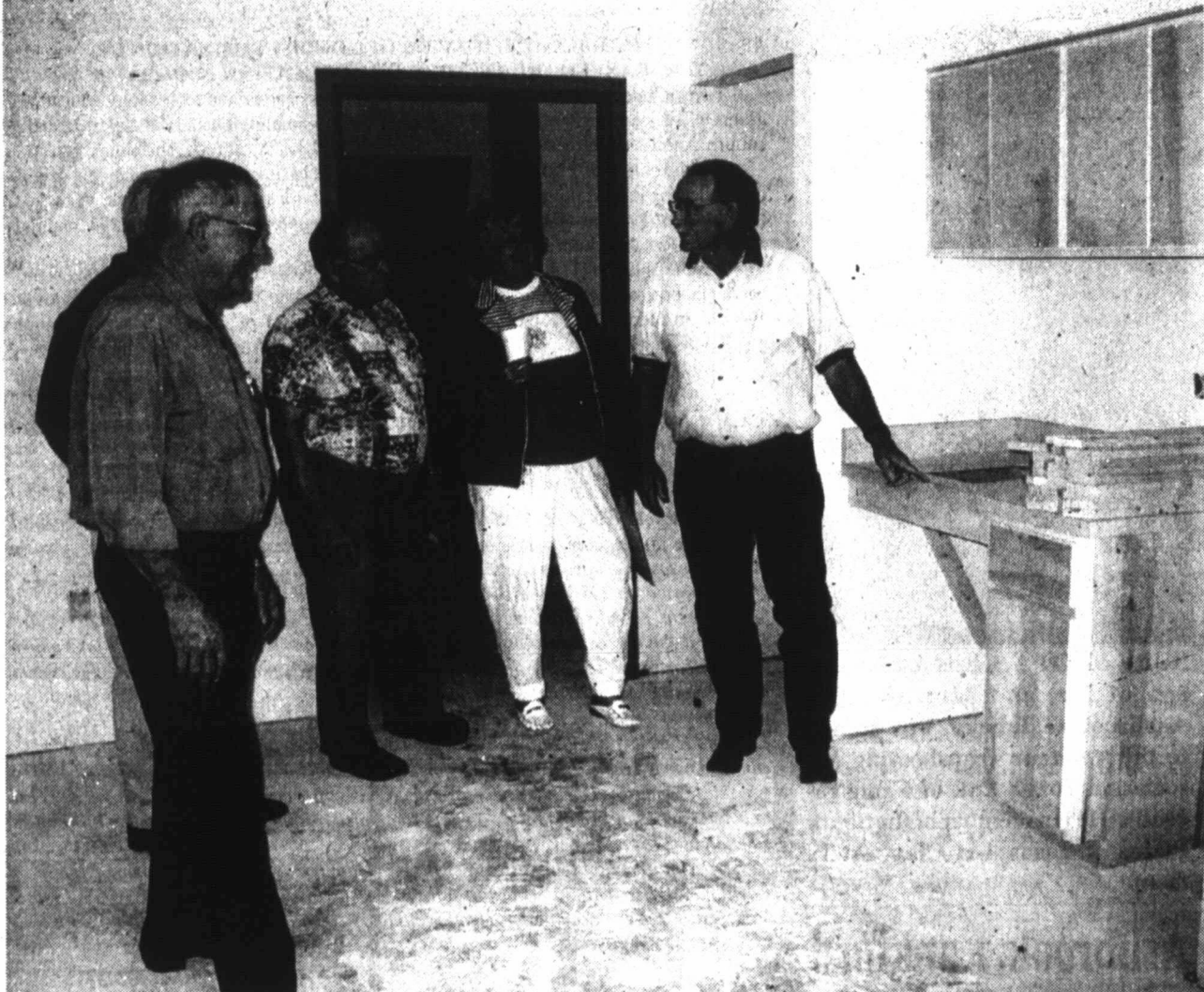
THE SINK GOES HERE - Lynn County Hospital District Board President Billy Tomlinson (right) seems to be pointing to the location of a sink in one of the apartment units as hospital directors toured construction progress at Lynnwood Assisted Living Center following the monthly board meeting last Wednesday. Construction is progressing on the 20-unit facility, but opening date has been delayed to mid-September or later, according to Hospital Administrator Dan Powers, who took hospital directors on the tour. Shown from left are directors Jerry Ford, Dalton Wood and Joan Knox, with Powers standing behind Ford. (LCN PHOTO)
