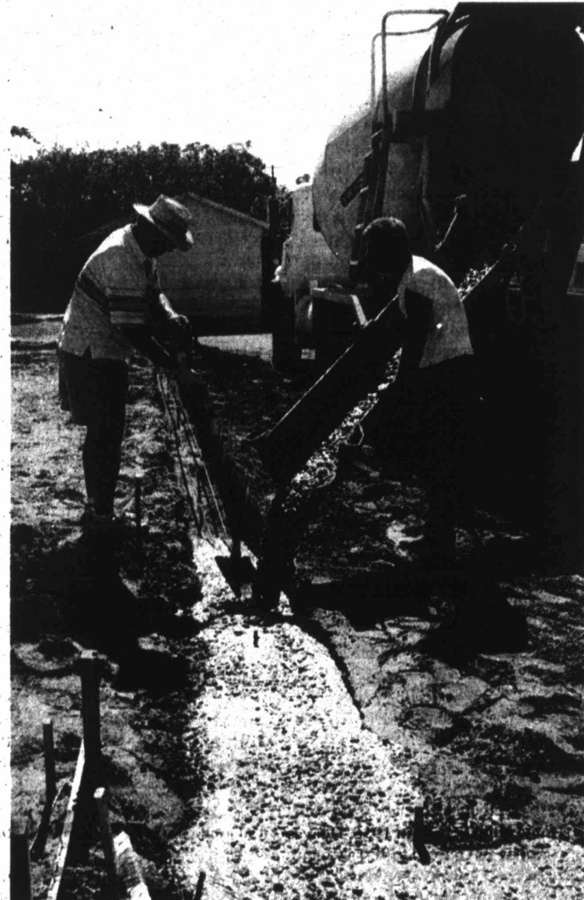
WORKING TOGETHER - Tahoka Trinity Church members Charlie Mac Holland and Phillip Barnett guide the concrete into the perimeter footing for a new church building at a workday last Saturday. An old fashioned "church raising" is scheduled in the near future, with the church being built from volunteer labor - something almost unheard of in this day and age. (LCN PHOTO)
