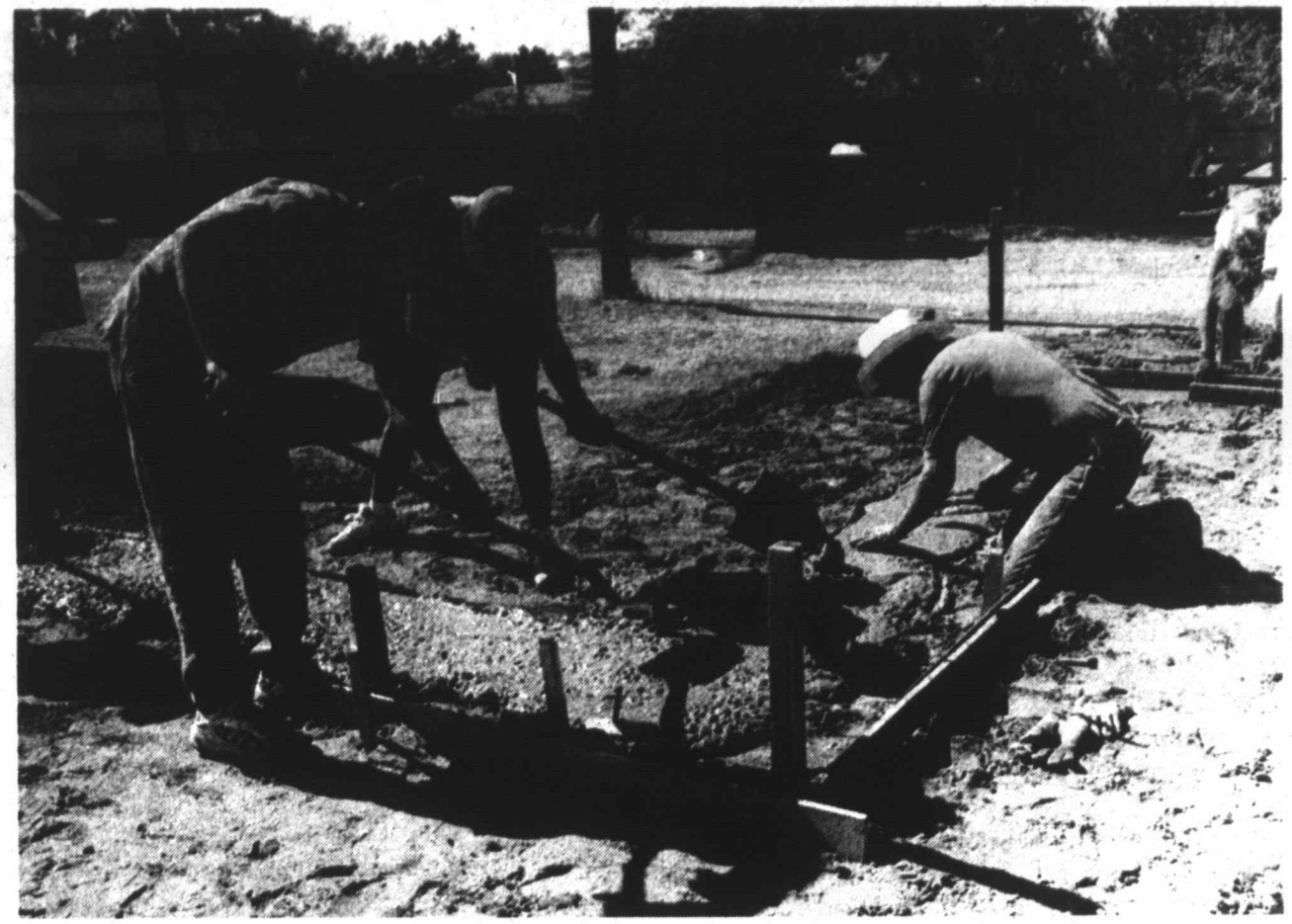
HANDS OF FAITH - Tahoka Trinity Church pastor Charlie Stice (kneeling right) works with Timmy Stice and Toy Holland Saturday morning as church members gathered to put their faith to work. The members of the congregation are volunteering their labor in building a new church, located directly behind their current facilities at 1925 Lockwood. (LCN PHOTO)
