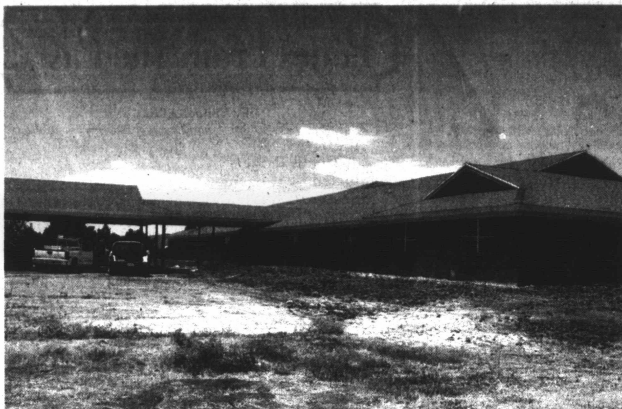
LYNNWOOD CENTER PROGRESS - Construction work progresses at the Lynnwood Assisted Living Center just north of the Lynn County Hospital District. Brickwork has been mostly completed on the building and interior work continues. The center is expected to open this fall. (LCN PHOTO)
