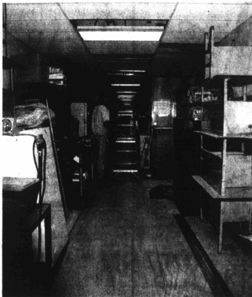
RENOVATION PROJECT - Desks and other paraphernalia were stacked high inside the hallways at Tahoka Elementary School as work continued on a renovation project this summer, including lowering ceilings to install ducts for the new heating/air system, new ceilings and lights, and new carpeting in much of the campus. Additionally, many rooms received a new coat of paint. The work is expected to be completed before students and teachers return in mid-August. (LCN PHOTO)
