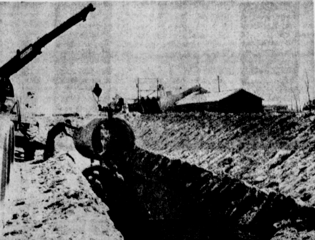
LAYING THE PIPELINE for Muleshoe's new storm sewer, workmen started on the east side of town and a week later had
