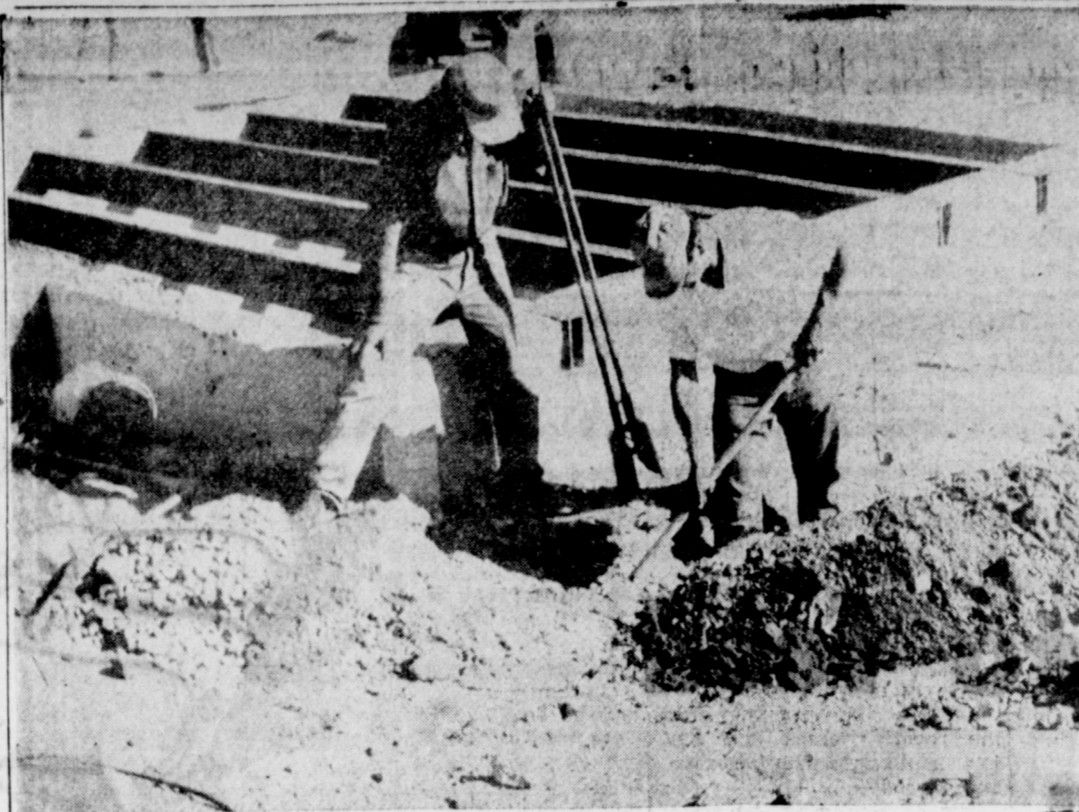
CONSTRUCTION WELL UNDERWAY — Co. Inc. Construction began June 10 on this elevator, which will bring Muleshoe 1 on the 500,000 bushel storage elevator under construction at Muleshoe Elevator bushels.
