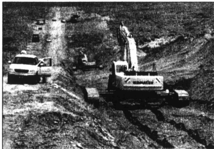
The extra-wide wheels on this excavator allows passage over the large ditch as the dirt is packed in over the finished pipeline. About 10 miles of the 31-mile pipeline has been completed.
