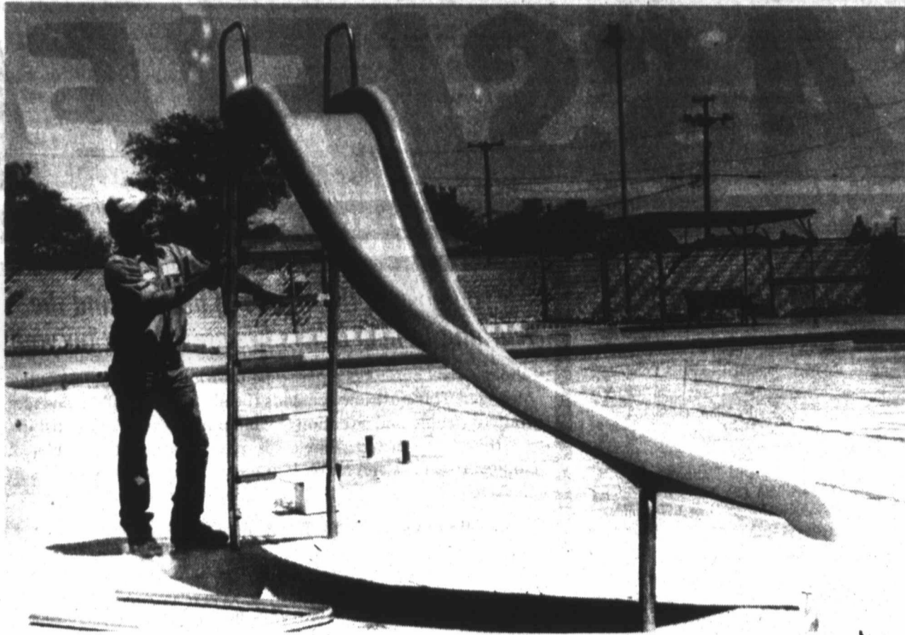
NEW WATER SLIDE - City employee Danny Moore eyes the new water slide which is being installed at the Tahoka City Pool this week in preparation for opening day (today). The high diving board has been lowered to a medium height for safety reasons, and the low diving board remains. The pool will be open Monday through Saturday, from 12:30-5:30 p.m. (LCN PHOTO)
