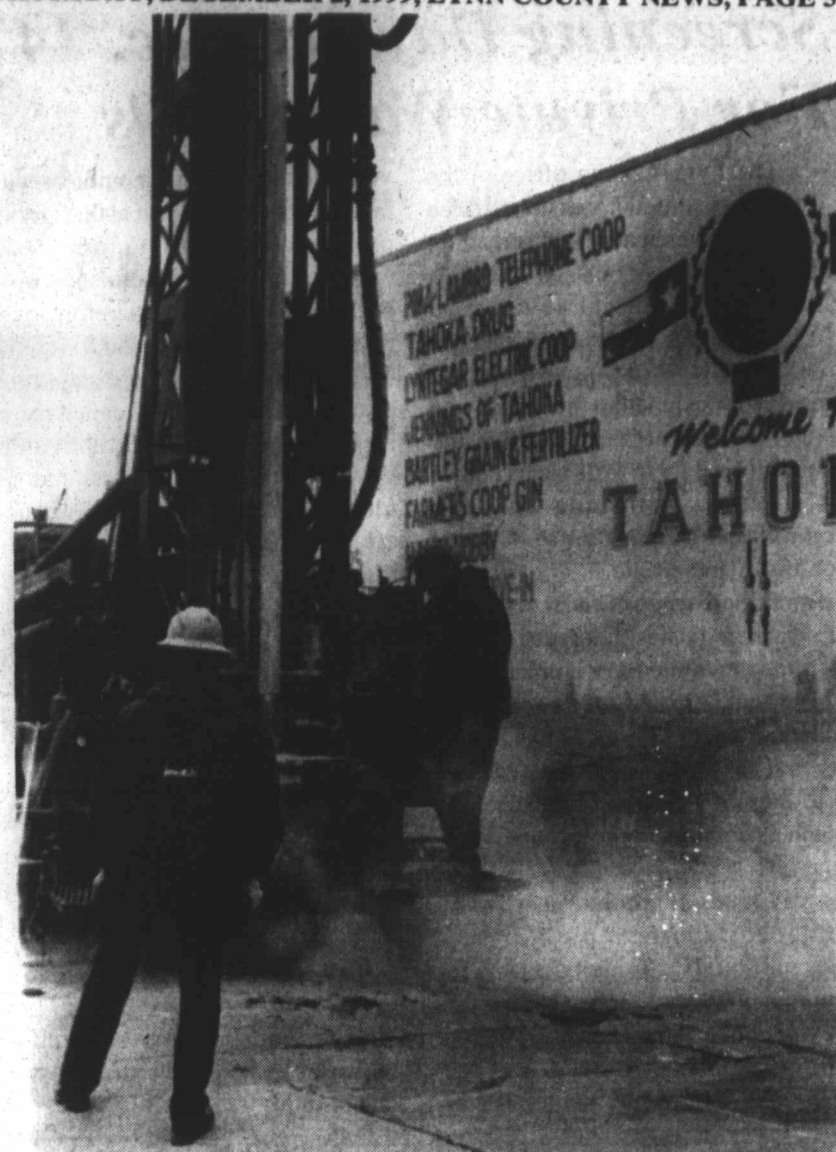
TESTING SOIL SAMPLES - Folks downtown were curious as they saw drilling in several locations this week, including this site next to the Lynn County News. Drilling down 65 feet, the workers were taking soil samples for testing contaminants from underground gasoline tanks in nearby locations. News Office staff were hoping for "bubbling crude and a trip to Beverly" but dust was all that came up. (LCN PHOTO)
