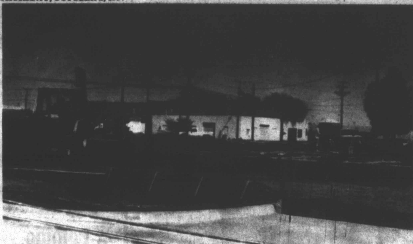
EARLY CONSTRUCTION PHASE - Construction has begun on the corner of Ave. K and S. 3rd for the Tahoka Housing Authority's new office/community center complex. The 6,040 sq. ft. facility will house office and boardroom facilities for the Housing Authority, as well as a community room, kitchen, and two smaller classrooms. In this photo, workers prepare the site for the foundation, which is expected to be poured next week. (LCN PHOTO)
