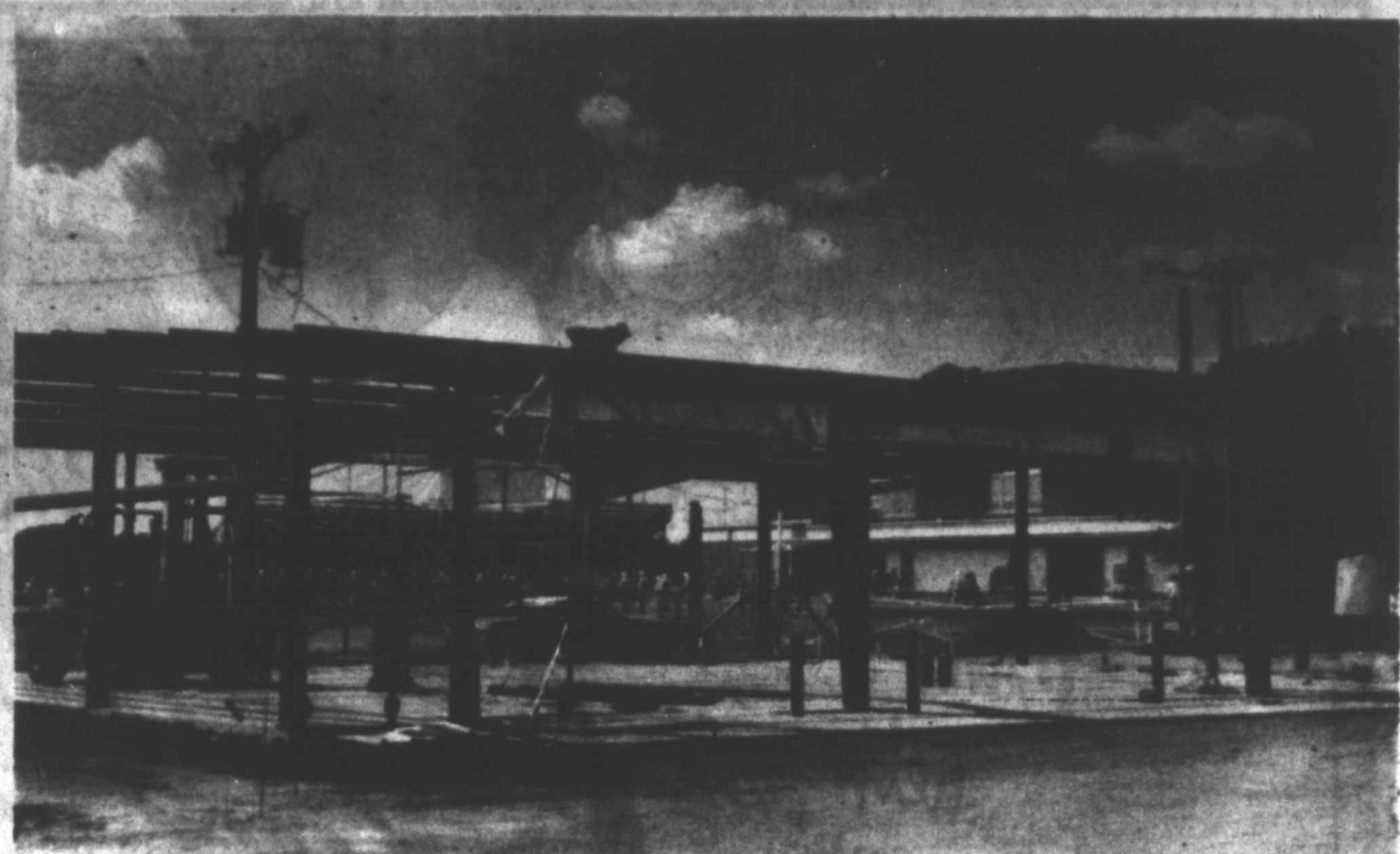
FRAMEWORK GOES UP - The metal framework for the new ag shop complex at the Tahoka High School campus went up this week, as workers continued on the project. The metal/brick building will house a new ag classroom and workshop, as well as a small office and bathroom facilities. (LCN PHOTO)
