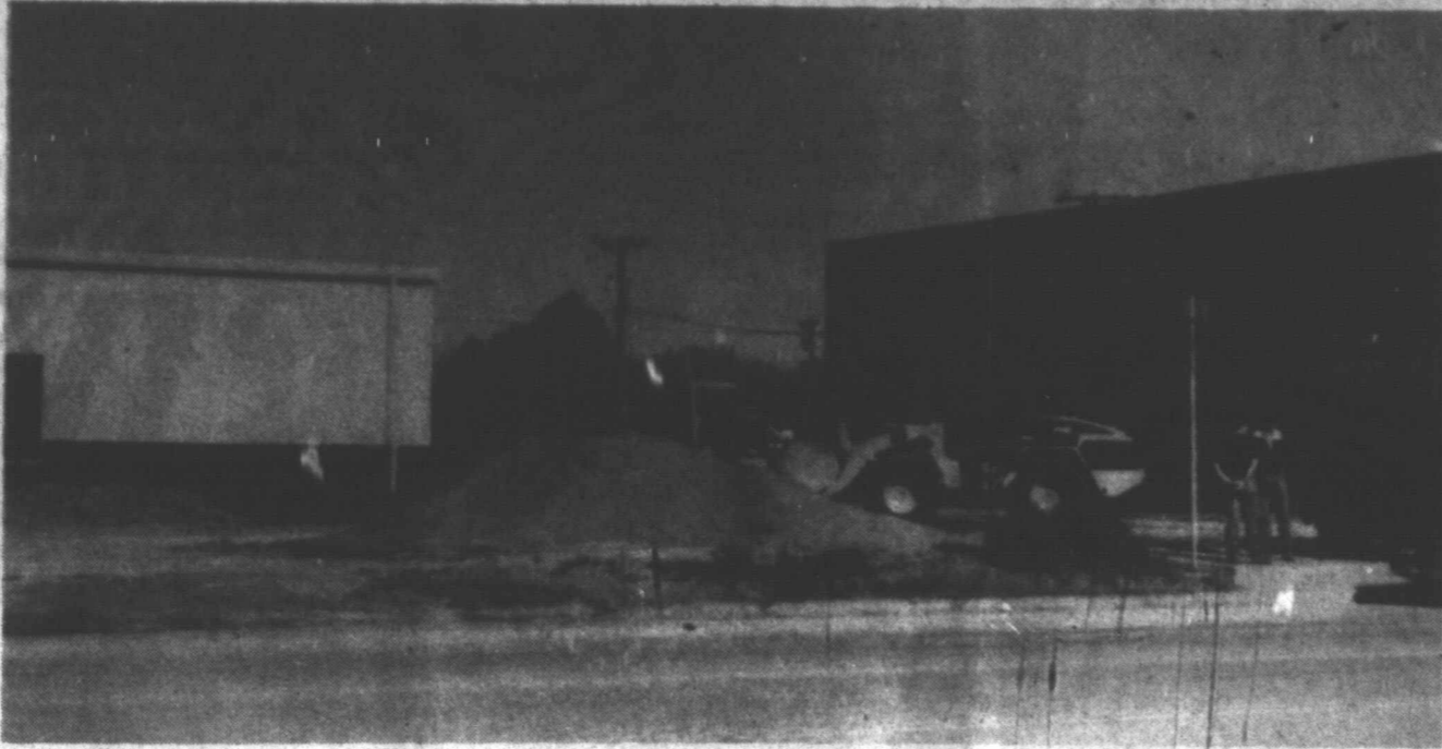
LANDSCAPE WORK BEGINS - Lynn County Commissioner Mike Braddock looks on (right) as county workers use precinct equipment to level the ground at the new Life Enrichment Center in Tahoka. Commissioners offered county assistance in the $219,000+ city project which has been funded entirely with donations from private foundations and area businesses, organizations and individuals. The construction phase is nearing completion as landscaping work begins this week. A ribbon cutting ceremony for the new center is being planned for June 21. (LCN PHOTO)
