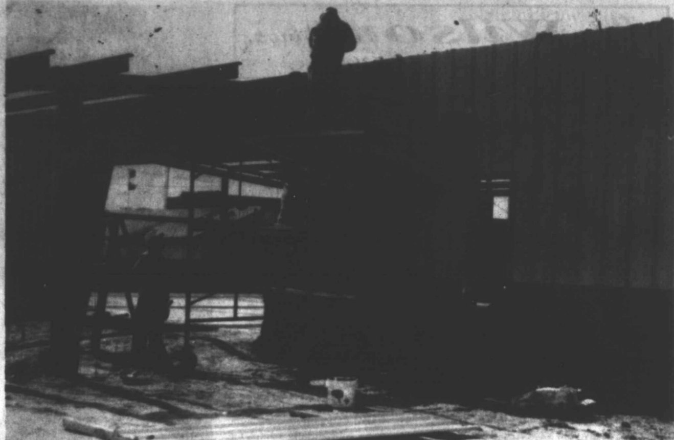
NEW LIFE ENRICHMENT CENTER - Progress continues this week on the new Life Enrichment Center for Tahoka and the surrounding area. In this photo, taken Monday, the walls were being erected. Tim Walker, general contractor for the building, invites area residents to a community meeting on Tuesday, Feb. 25, at 5:30 p.m. at Tahoka City Hall, where he will answer any questions regarding the construction of the facility. (LCN PHOTO)
