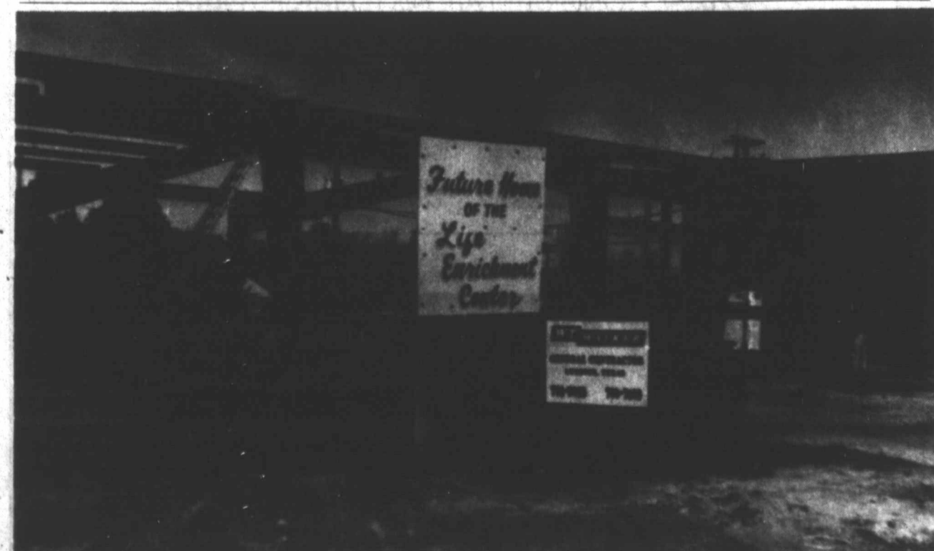
PROGRESS — Construction work is progressing on the new Life Enrichment Center on Main Street in Tahoka. This photo was taken Tuesday as the framework was put into place. Completion of the project is expected within six months. (LCN PHOTO)
