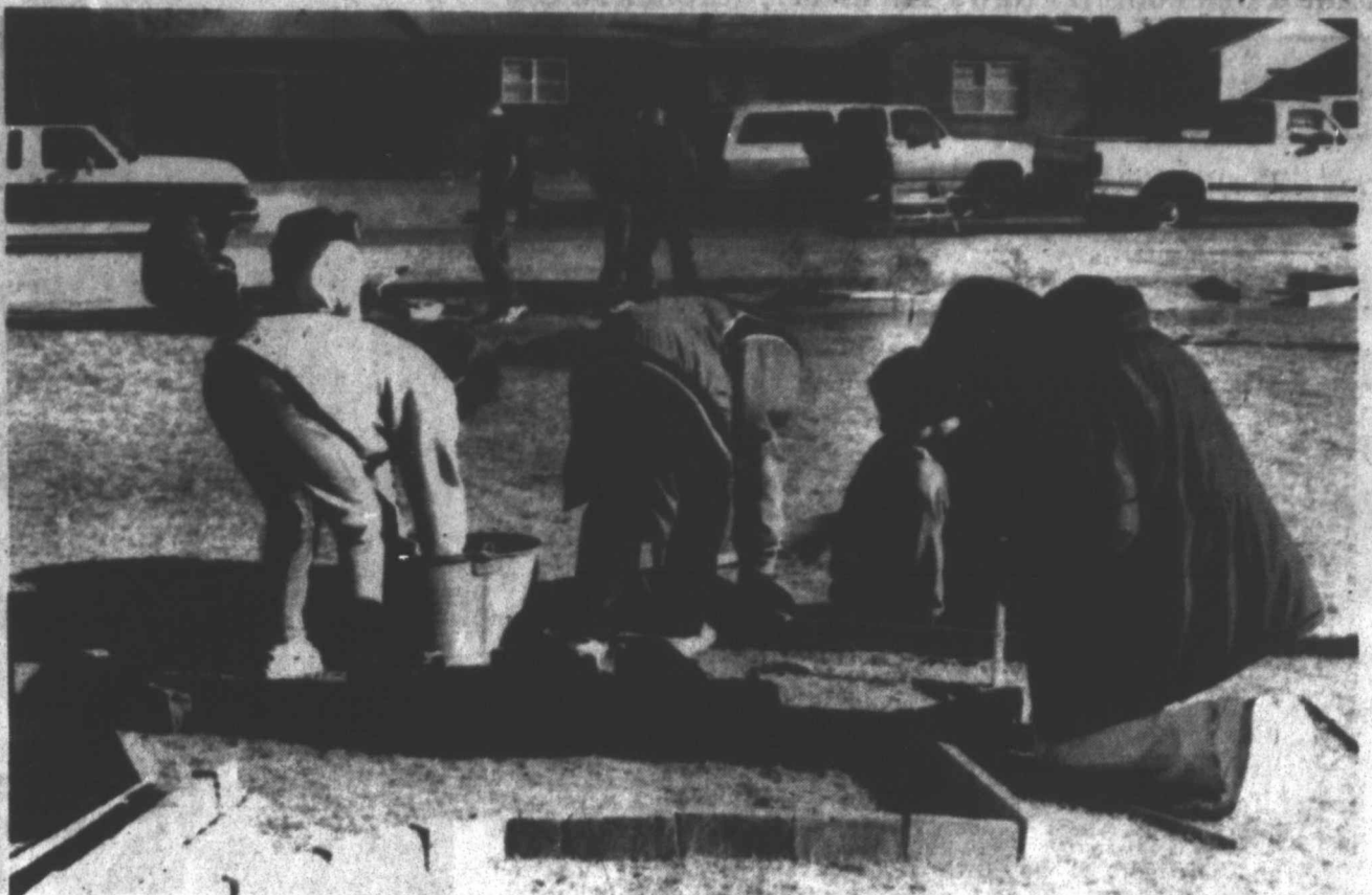
WORKING HARD - These Tahoka Middle School youth are hard at work building their miniature golf course hole, called Giant Texas Star, last Friday, when seventh and eighth grade students teamed up with a dad for the morning project. Shown here is Marvin Gregory (right) with his team, including daughter Carrie, Michael Farrell, Luz Mendez, Raul Garza and Adrian Garcia. (LCN PHOTO)
