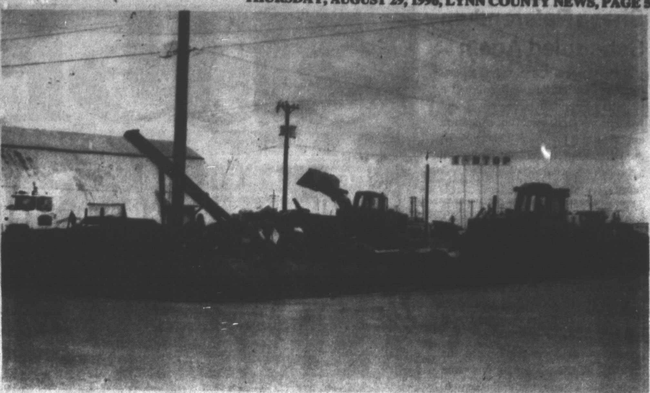
LOT BEING RAZED - Workers began this week clearing the lot on Hwy. 380 just west of the Hwy. 87 west access road, in preparation for a new Town & Country store which is going to be built here. (LCN PHOTO)
