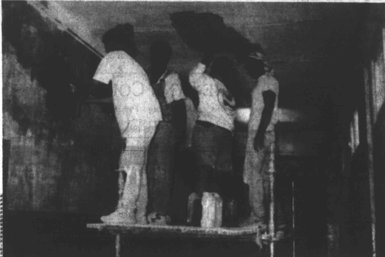
HARD AT WORK - Terri Solomon (second from right) rolls primer onto the ceiling at the Istra Children's Home in Russia, assisted by her college friends from the Texas Tech Wesley Foundation, (from left) Cindy Gassiot (formerly of Tahoka), Jen Ahrnes and Daniel Mayberry. A group of 10 college youth spent two weeks on the Russian mission trip, working on repairing the walls and spending time with the children there.
