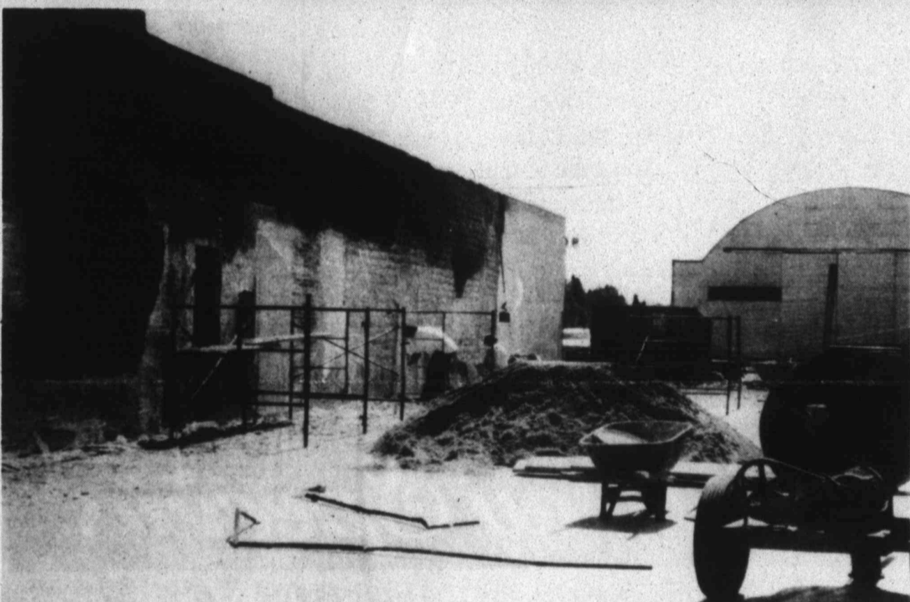
CLEANUP CONTINUES DOWNTOWN - Workers this week continued to clean up debris and repair walls of the building next door to the Tumbleweed Cafe which burned following an explosion on May 8. Michael McKean, owner of the cafe, was charged last week with arson in the fire which left the restaurant on Main St. in downtown Tahoka a pile of rubble. This photo of the area just north of the Tumbleweed is where a vacant building stood, also destroyed in the fire. The owner of the building housing the restaurant has yet to begin cleaning up the pile of charred rubble there. (LCN PHOTO)
