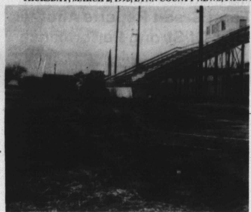
WORK BEGINS ON NEW TRACK — Work began this week on the new Tahoka High School track at the football field as bulldozers prepare the foundation. Most of the construction work is expected to take place in March and April. The school district contracted with Armor Asphalt, a Lubbock firm, for the seven-lane track. (LCN PHOTO)
