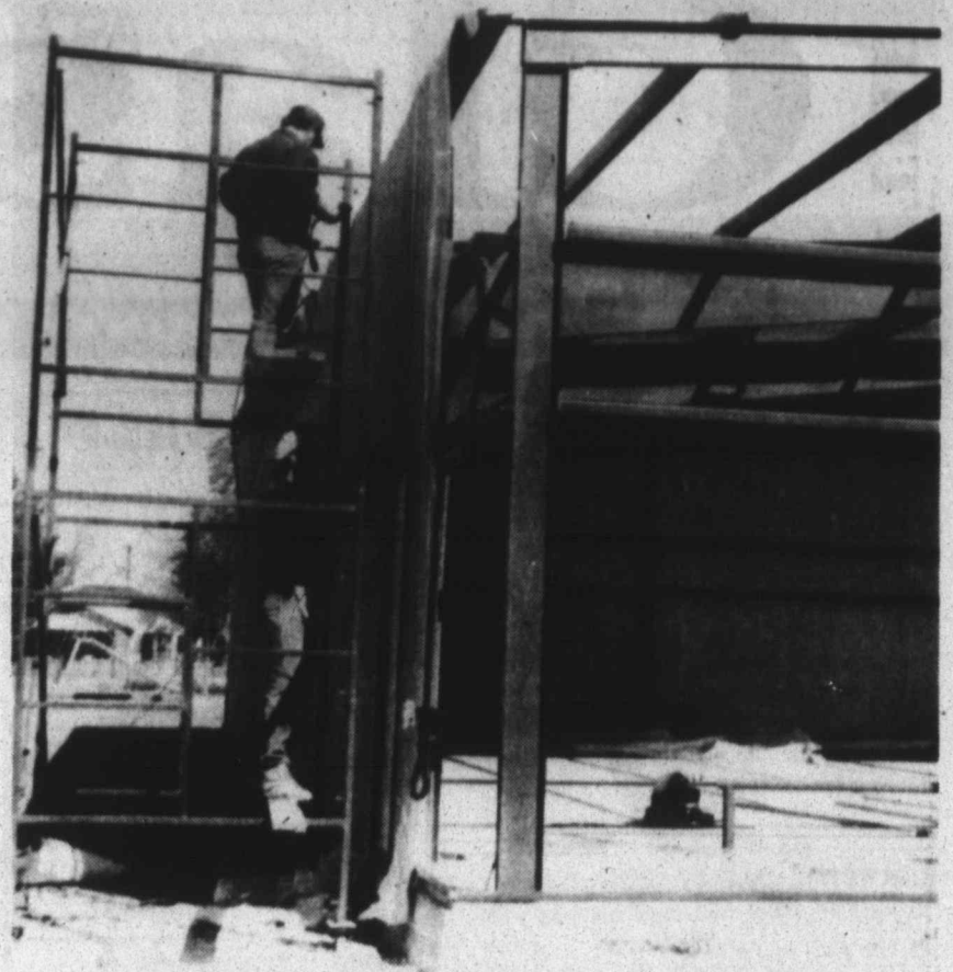
WORK PROGRESSES -- Work continues this week on the new Tahoka Fire Hall as insulation and siding are installed.
