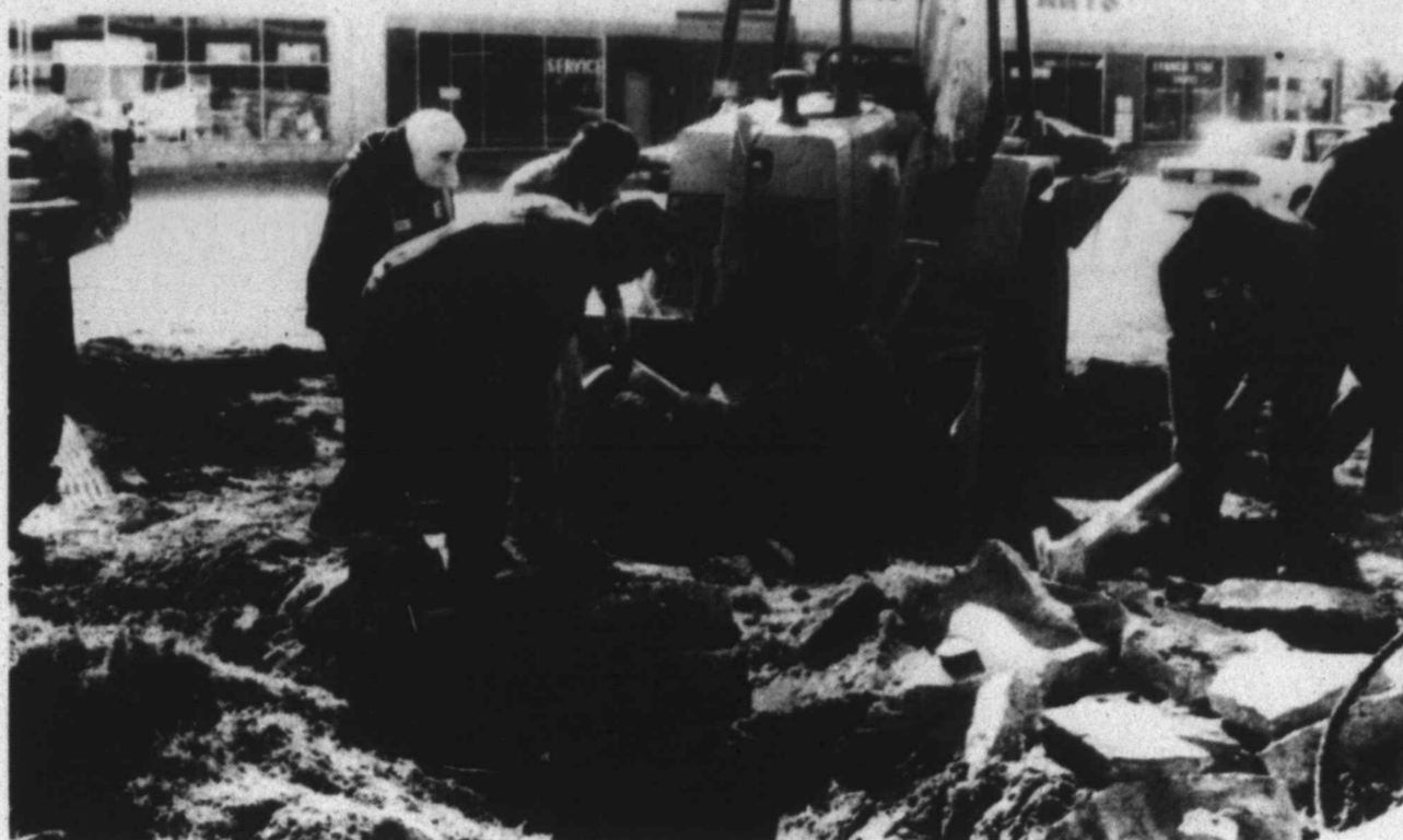
BREAKING GROUND FOR NEW FIRE HALL - City of Tahoka workers Tuesday began preparing the site for the new fire hall which will be constructed adjacent to City Hall. The Town Crier marquee has been temporarily removed until it can be relocated to another site near City Hall. (LCN PHOTO)
