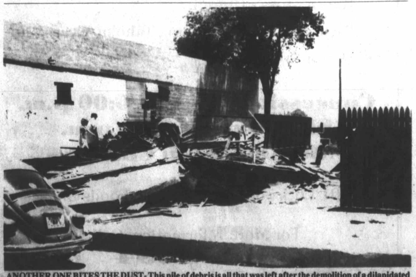
ANOTHER ONE BITES THE DUST- This pile of debris is all that was left after the demolition of a dilapidated building in downtown Tahoka. Complying with a strict new city ordinance, owners of the building at 1511 S. 2nd had the building (many years ago an army surplus store) demolished and, shown here, the debris hauled off. Several other buildings in Tahoka have been targeted by the ordinance, and city officials expect owners to comply or face court proceedings. (LCN PHOTO)
