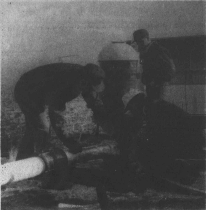
NEW HYDRANT DEMONSTRATION - Tahoka Volunteer Firemen Bruce Horwood, left, and Wesley Boone, right, hook up a fire hose to the new dry hydrant located approximately 14 miles north of Tahoka on Hwy. 87, just inside the county line. Fire Chief Steve Miller looks on. The new design facilitates water access to irrigation wells for rural fire departments, and is being eyed with interest by the Texas Forest Service, who funded the venture through the Wes-Tex RC&D here.
