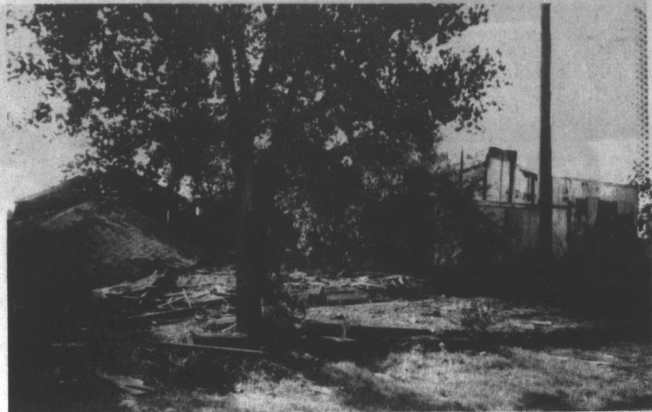
BUILDING GOES DOWN—A dilapidated building on Ave. H near Lynn County jail was torn down last week.
