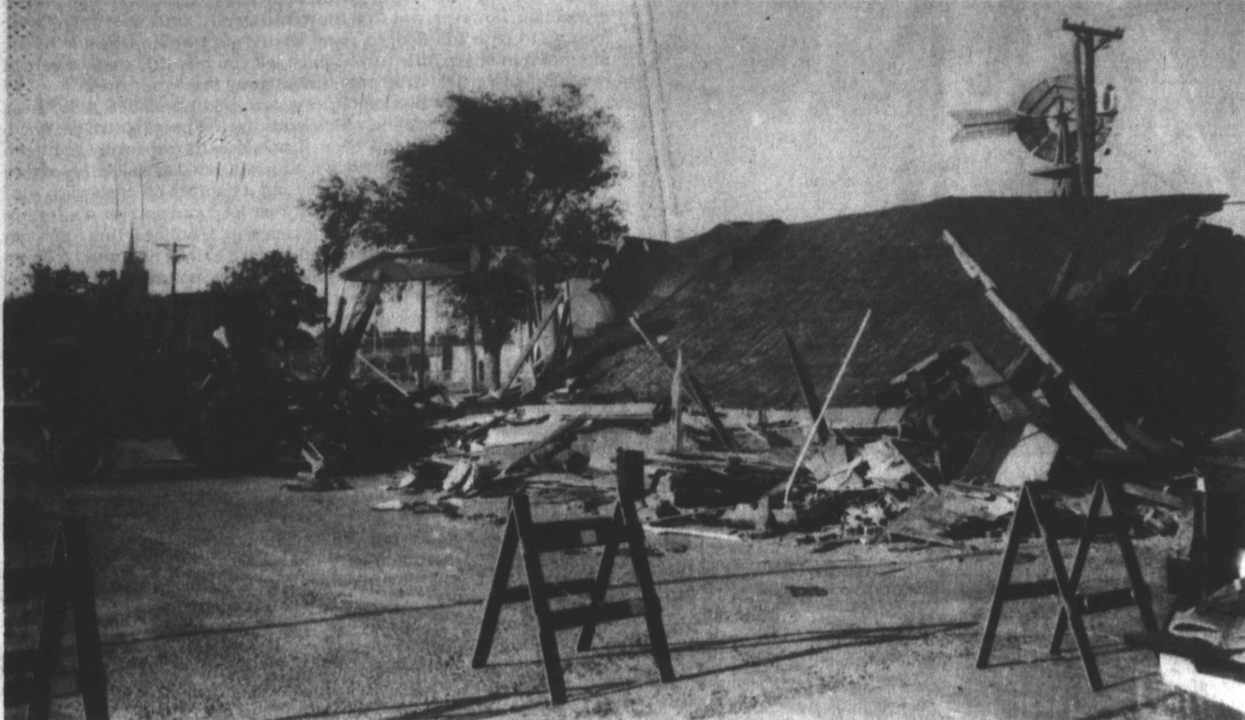
SCOUT HUT GOES DOWN —No, the Scouts didn't get out of hand at the last meeting in the Scout Hut next to Tahoka City Hall. The city contracted to have the old building demolished, and workers did just that over the weekend. (LYNN COUNTY NEWS PHOTO by Warren Hardt III)
