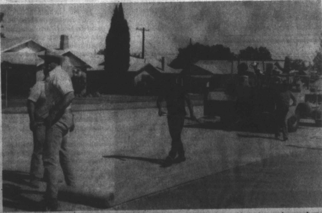
SEAL-COATING IN CITY—Workers for Zahn Construction Co. of Lubbock this week wound up work on seal-coating streets in Tahoka, mostly in the northwest section of the city. (LYNN COUNTY NEWS PHOTO)
