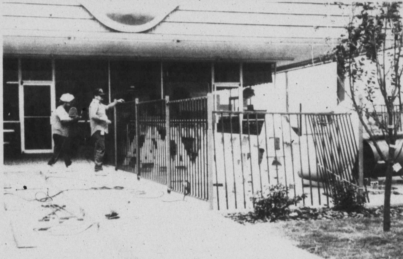
FACE-LIFTING AT THE DQ—Tahoka Dairy Queen, under new ownership, last week was undergoing some remodeling outside, where playground equipment was being installed. The Dairy Queen already has added some new outside tables and seats. (LYNN COUNTY NEWS PHOTO)
