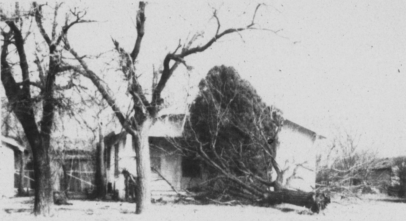
WIND DAMAGE—High winds last Thursday uprooted this tree on the southeast corner of Main and 7th St. in Tahoka. The home is owned by Tom Cloe. The wind gusted to 65 that day. (LYNN COUNTY NEWS PHOTC)
