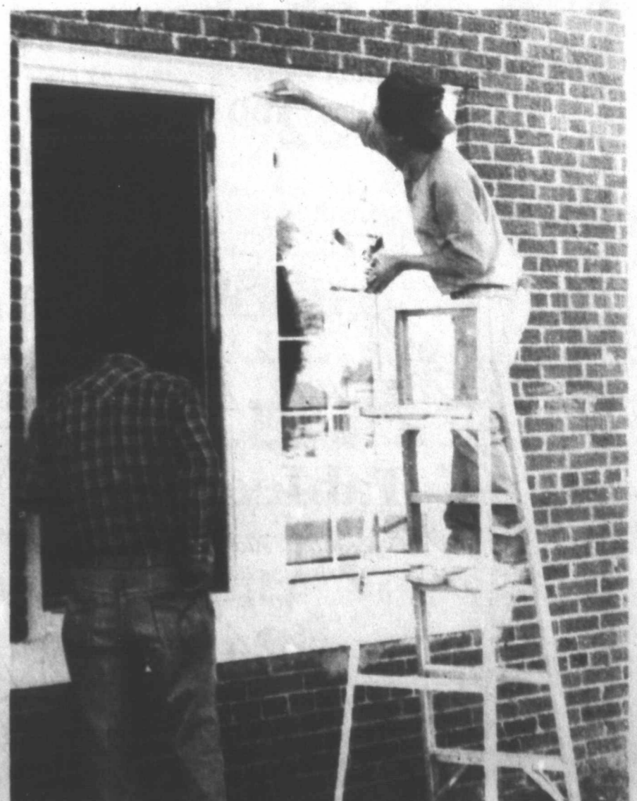
GETTING A NEW LOOK—Windows on the ground floor of the old Keltner Hotel are being replaced as work is underway on renovating the facility in Tahoka as quarters for the South Plains Community Action operations in Tahoka.
