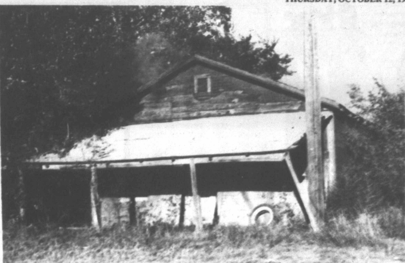
DAMAGED BY FIRE —This unoccupied house on Ave. H just south of Taylor Tractor and Equipment Co. was damaged by fire about 5:30 p.m. Tuesday. Smoke can be seen coming from the attic area. Tahoka volunteer firemen were working on the other side of the building to stop the fire.
