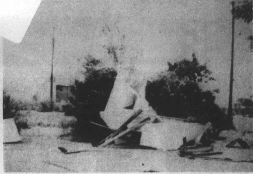
STORM DAMAGE — This storage shed at the home of John Chapa Jr. on South 3rd Street was blown apart by high winds during the rain storm Tuesday evening.
