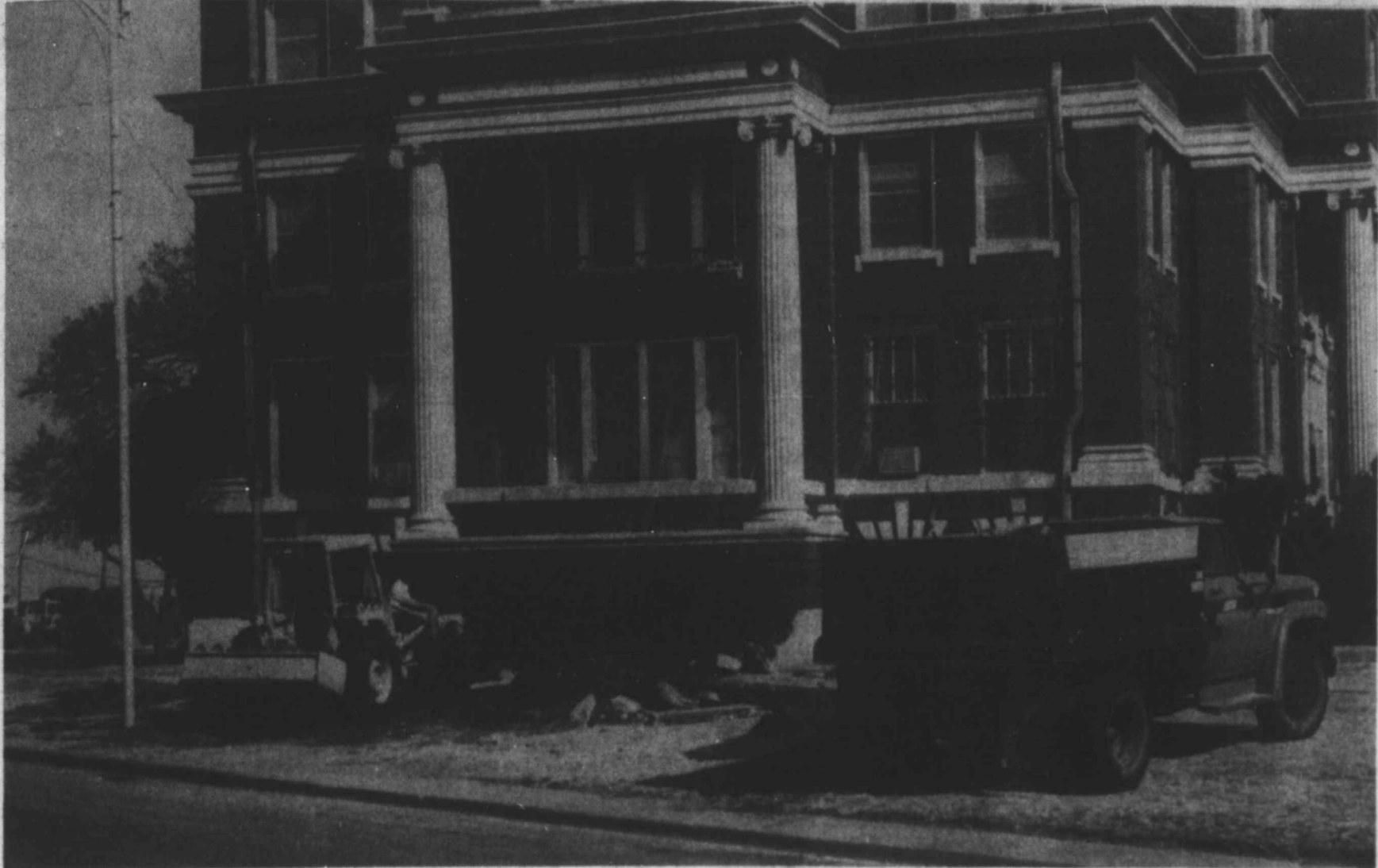
COURTHOUSE WORK STARTS — Work started last week on remodeling the basement of the courthouse in Tahoka, including construction of a ramp on the west side of the building to make access easier for handicapped persons. Wardroup Construction Co. of Lubbock is contractor for the project. (LYNN COUNTY NEWS PHOTO)
