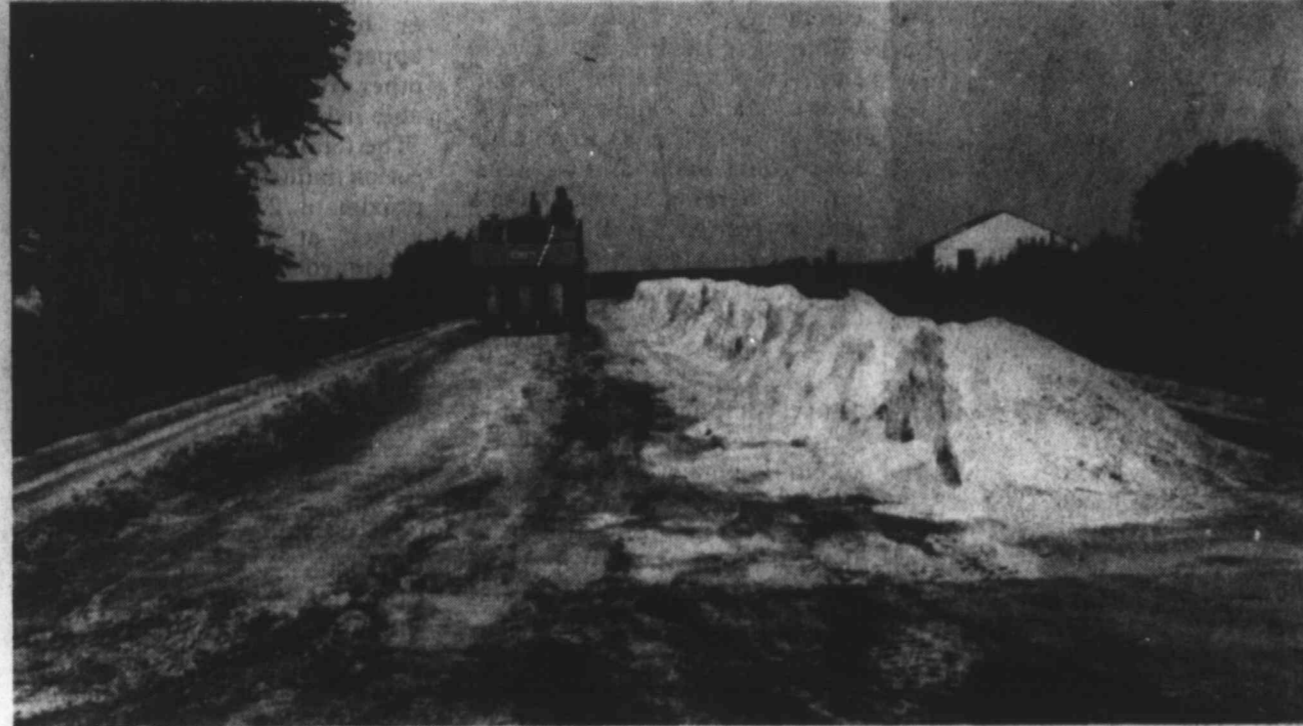
STREET WORK —Workers for Zahn Construction Co. of Lubbock were busy on this section of S. 3rd St. this week, part of the paving program in the city under the Community Development Block Grant plan. (LYNN COUNTY NEWS PHOTO)
