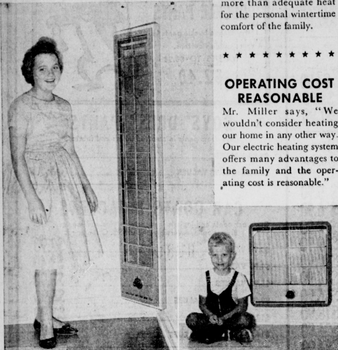
"Independent room control" is feature of electric heating system at H. H. Miller farm, Dawn, Texas. Radiant glass panels make attractive and safe installation and give exact degree of heating desired.
