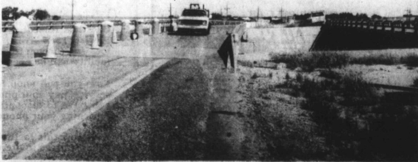
CONSTRUCTION REPAIR ON LYNN COUNTY BRIDGES UNDERWAY —Repair work consisting of installation of sealed expansion joints, two course surface treatments and asphaltic concrete pavement on five Lynn County bridges is underway due to damage from inclement weather this past winter. Amarillo Roads, Inc. is the contractor for the project. The bridge shown above is on U.S. 87 and Station 1742. (LYNN COUNTY NEWS PHOTO)
