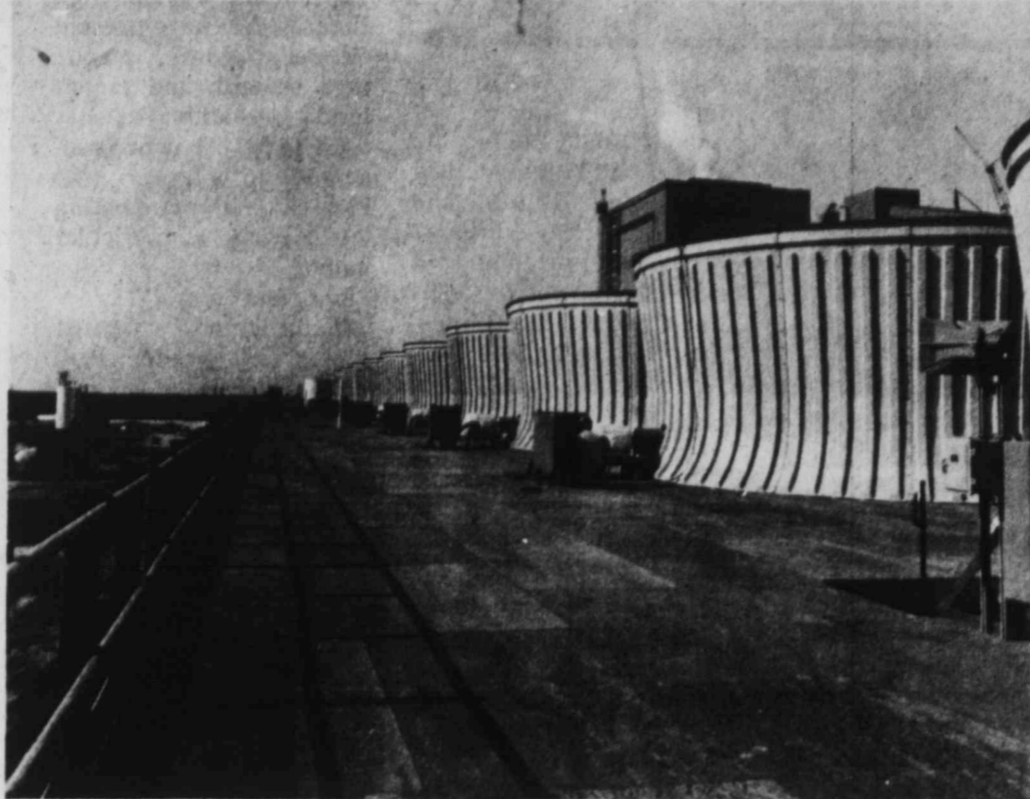
BIG COOLERS --A dozen giant fans pull air up through one of the two "cooling towers" at Southwestern Public Service Company's Tolk Station Unit No. 1. Each cooling tower works just as an evaporative cooler at a home does. The towers lower the temperature of water, which is used--and reused as many as five times--in the electricity-generating process at the coal-fired plant. (SPS PHOTO)
