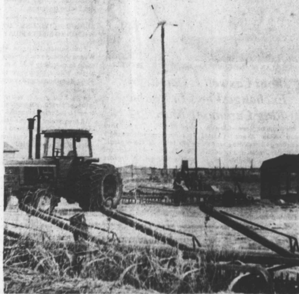
WHEN THE WIND BLOWS—the generator will gen. Winds such as the area suffered under Tuesday should make a lot of electricity with this wind-powered electric generator installed at the Kenneth Scott farm last week. Of course, when it gets over 40mph, the generator shuts off. The device is mounted atop a 54-foot pole. (LYNN COUNTY NEWS PHOTO)
