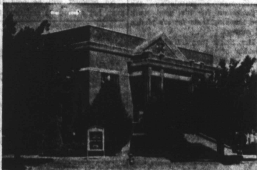
Tahoka residents cast their eyes upon the 40-year old First Methodist Church for the last time Tuesday. When the sun went down, the building no longer stood at the corner of North First and Ave. J. Wrecking crews, who have been dismantling the building, brought the walls down that day, making completion of the south wing of the new church possible.
