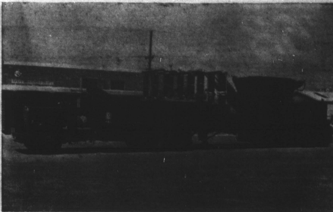
This is Southwestern Public Service Company's traveling transformer. The new unit, built to special specifications by General Electric, is designed to replace almost any transformer in the company's system in case of scheduled repair work or emergency. The transformer can be connected to any one of three voltages on the "high", or transmission line, side, or any one of five voltages on the "low", or distribution, side. The cost of the unit? $1.50 a pound, and it weighs 82,000 pounds.
